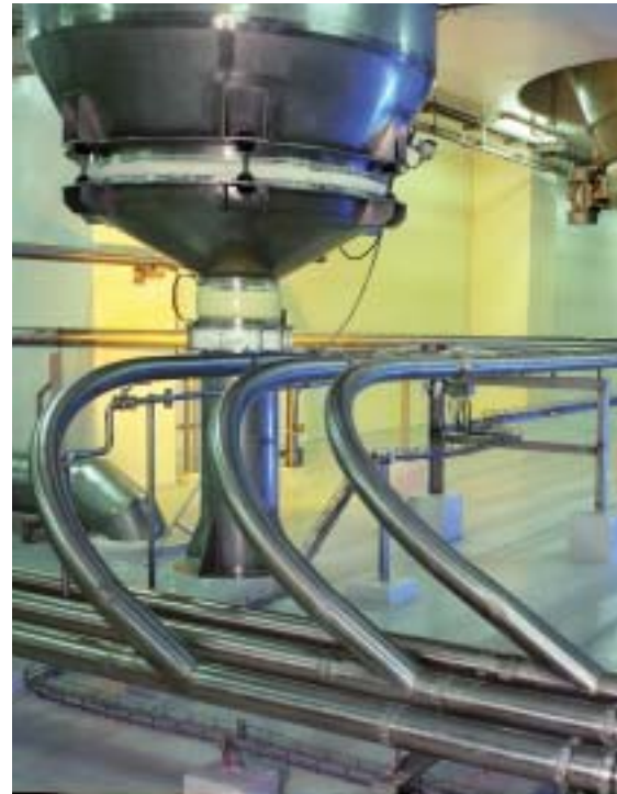
Bottom of powder silos. Pipelines connected for vacuum conveying product to bag filling machines
