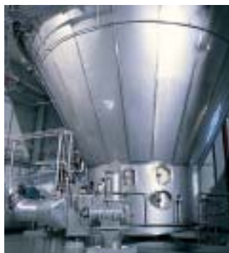
Conical part of CDP Dryer with powder outlet duct from the integrated fluid bed
